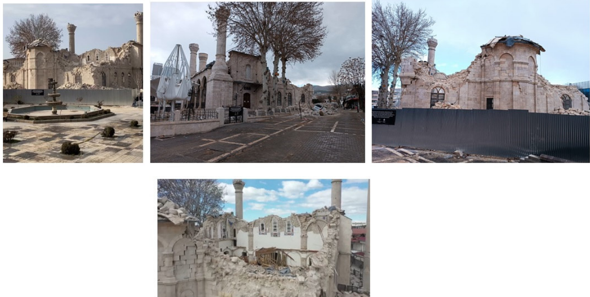
Figure 11. Views of the destruction of Yeni Mosque from different angles after the 6 February 2023 earthquakes (Author's archive)
